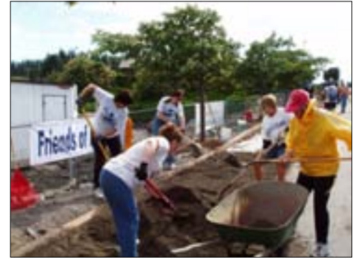
In June of 2006 approximately 60 FoF volunteers gathered for 3 days to clear sod, install wood curb and lay down 150' of crushed gravel walkway from just below the Post Office to the entry of the Payless parking lot.
